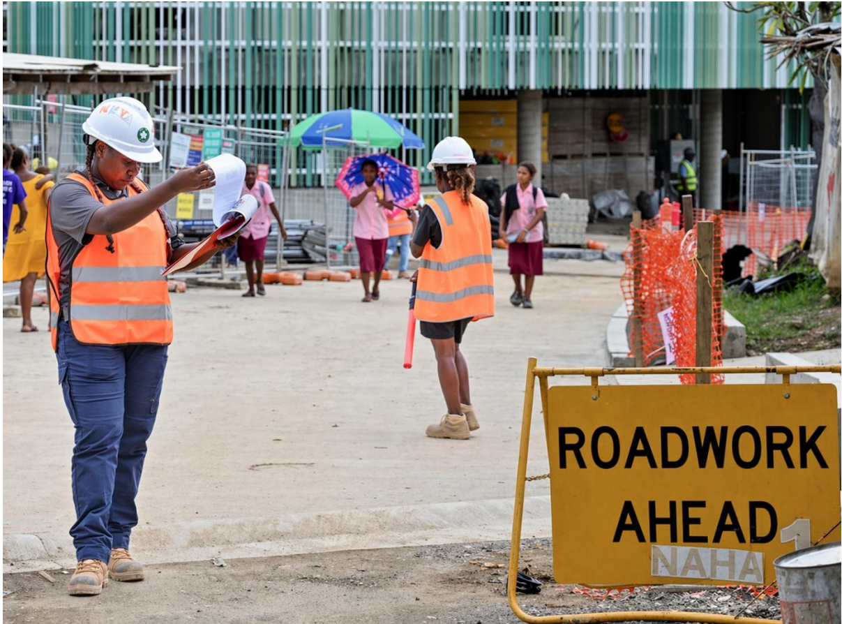
Photo 2 – Netania Tolinao reviews site safety plans at the Naha Birthing and Urban Health Centre project, helping to manage safe movement around active construction areas for both workers and the general public.
