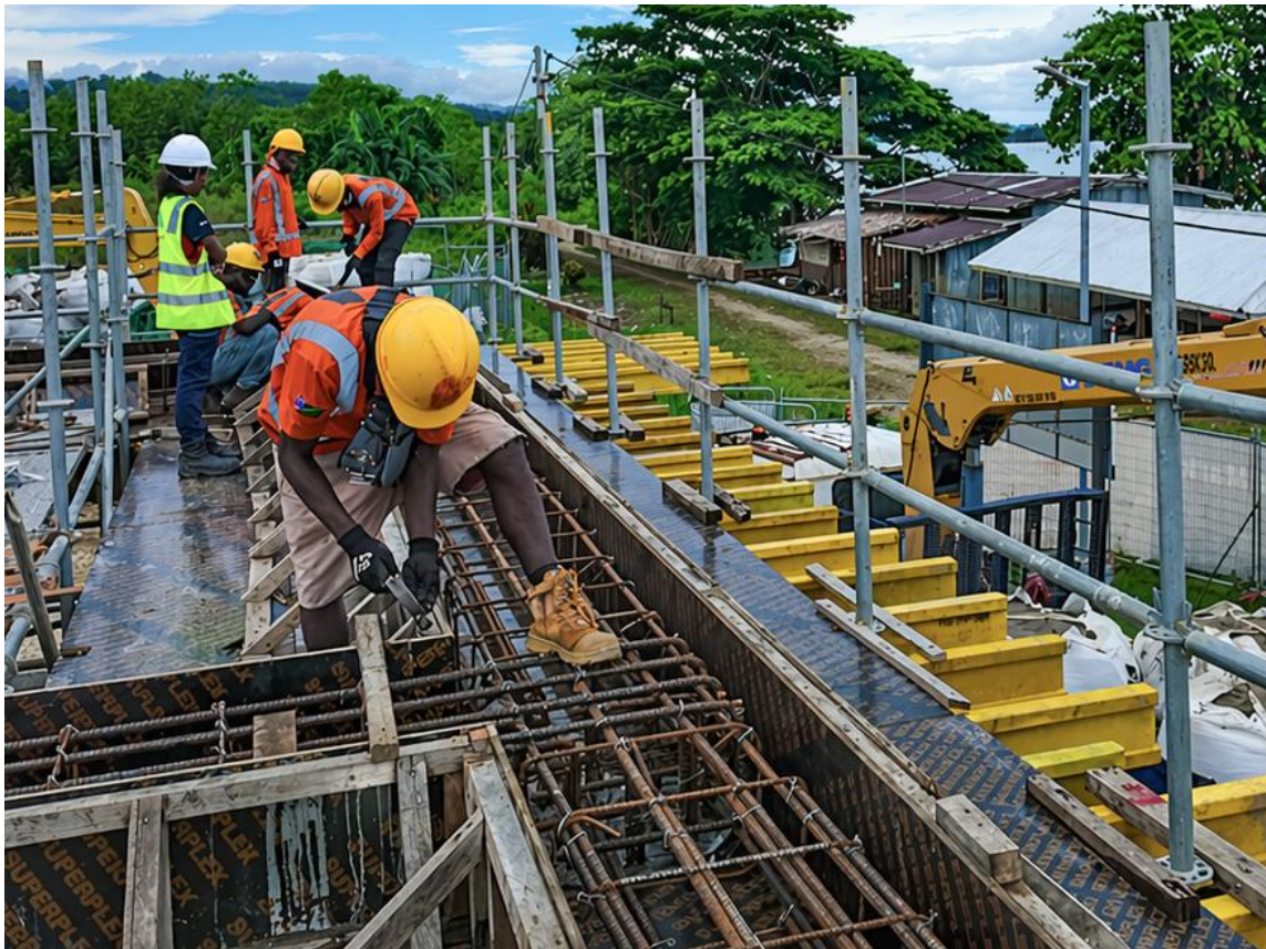
Photo 1 - Zitinah Rotu (far left) ensures a high standard of safety is met on the construction site of the new Seghe Market, Morovo.
